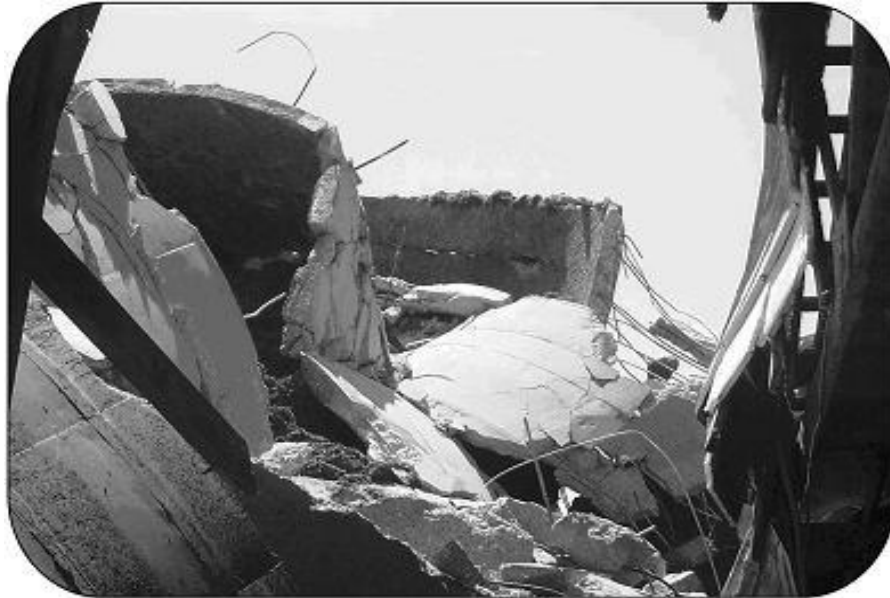
Fig10. Failure of silo due to earthquake
