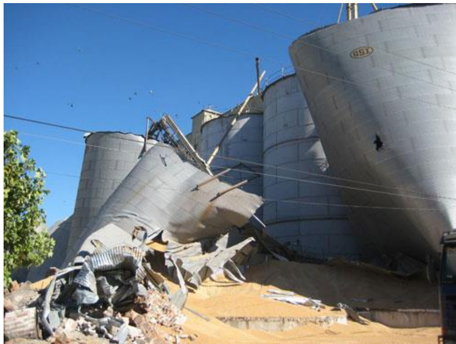
Fig.11 Failure of silo at segment 1 due to excessive stresses at junction
